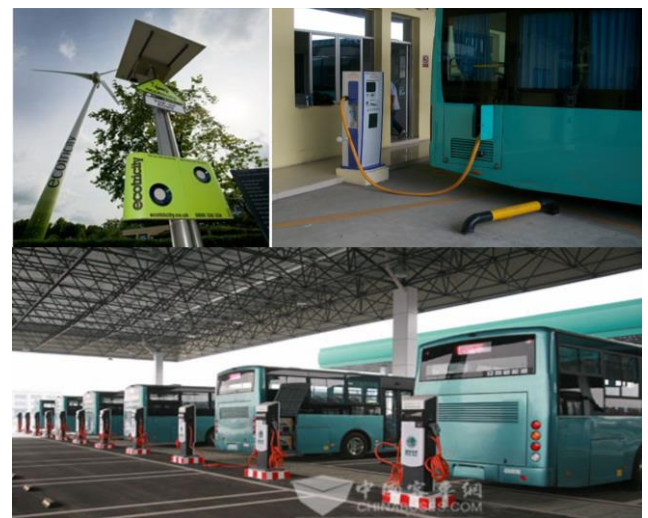
Figure 29: Images showing EV charging stations with charging pole, wind and solar panels
