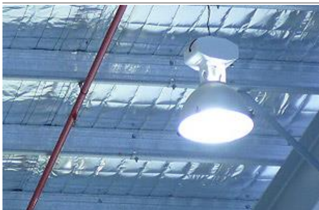
Figure 23: Lighting fixture in workshop
