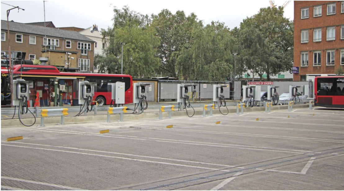
FIGURE 78: WATERLOO ELECTRIC BUS PARKING AND CHARGING INFRASTRUCTURE. SOURCE: (BUS&COACH BUYER, 2016)
